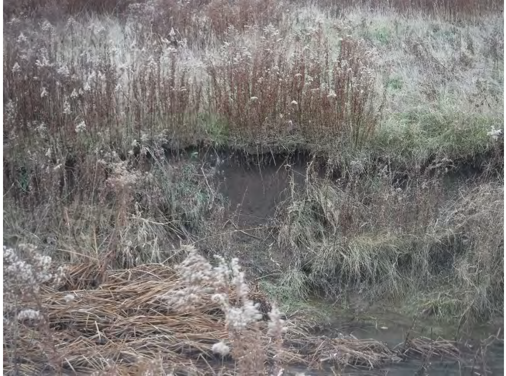
Photo 8: Typical evidence of recent bank erosion along Talbot Creek within the Study Area (facing east).
