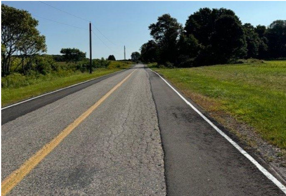
Substandard Ditching - Scotch Line west of Coon Road
