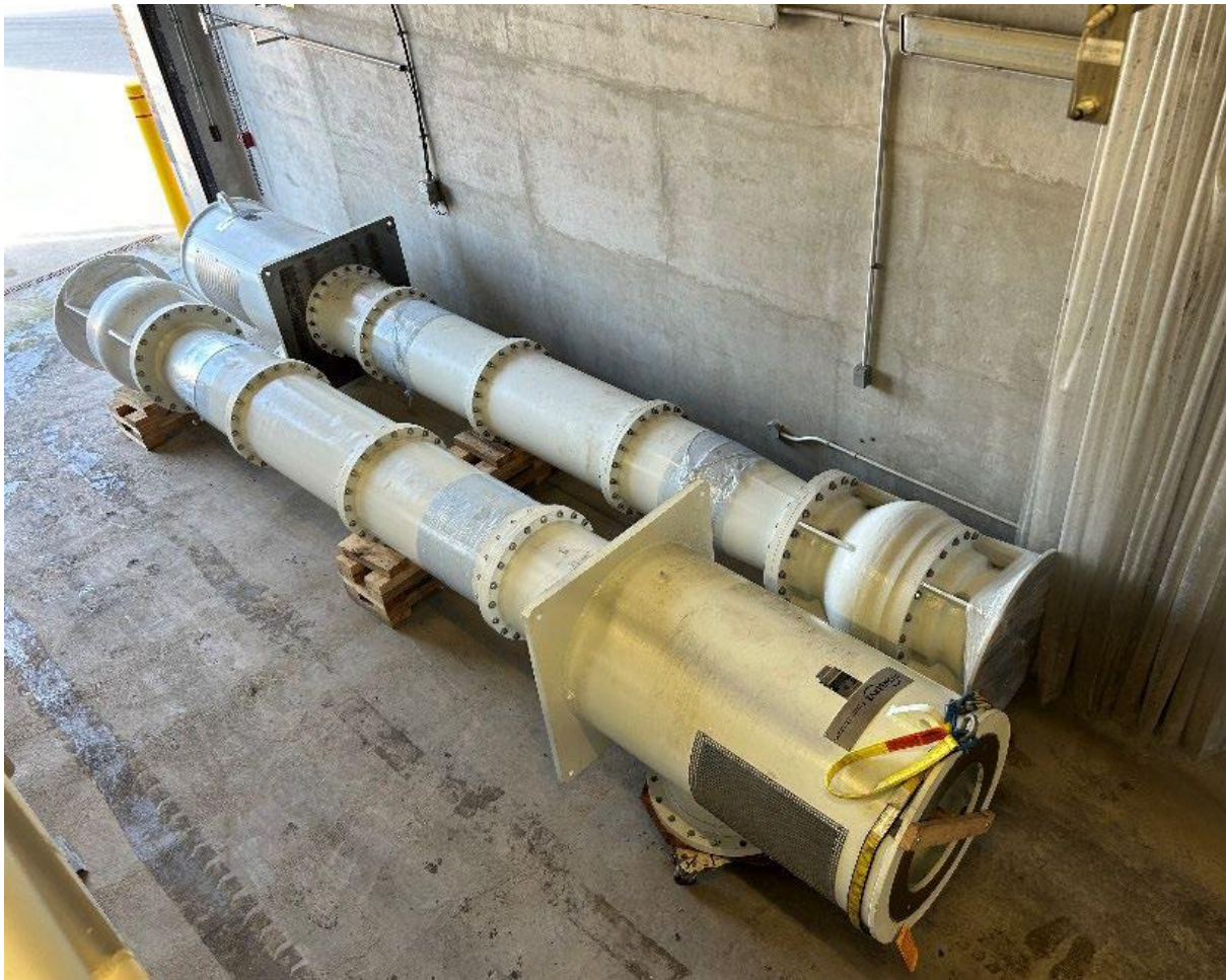
Figure 5: The new pumps delivered to the Elgin Area WTP in October 2024.
